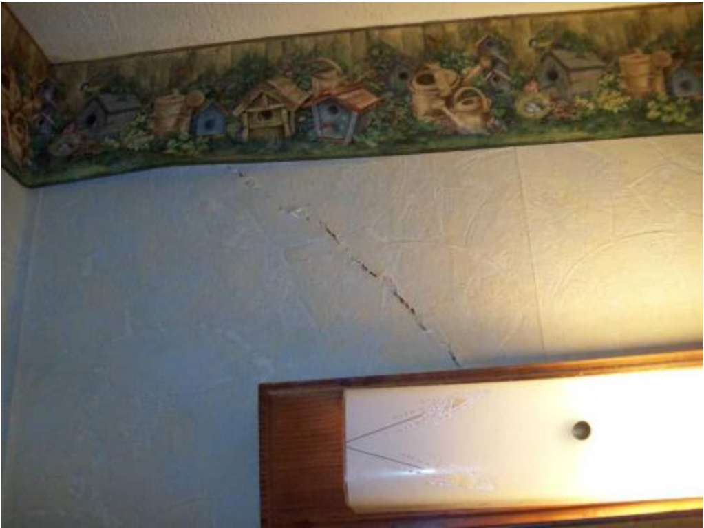
26 Master bath 7/18/2009 Taken By: Butch Bragg Additional damage from settlement in master bedroom bath
